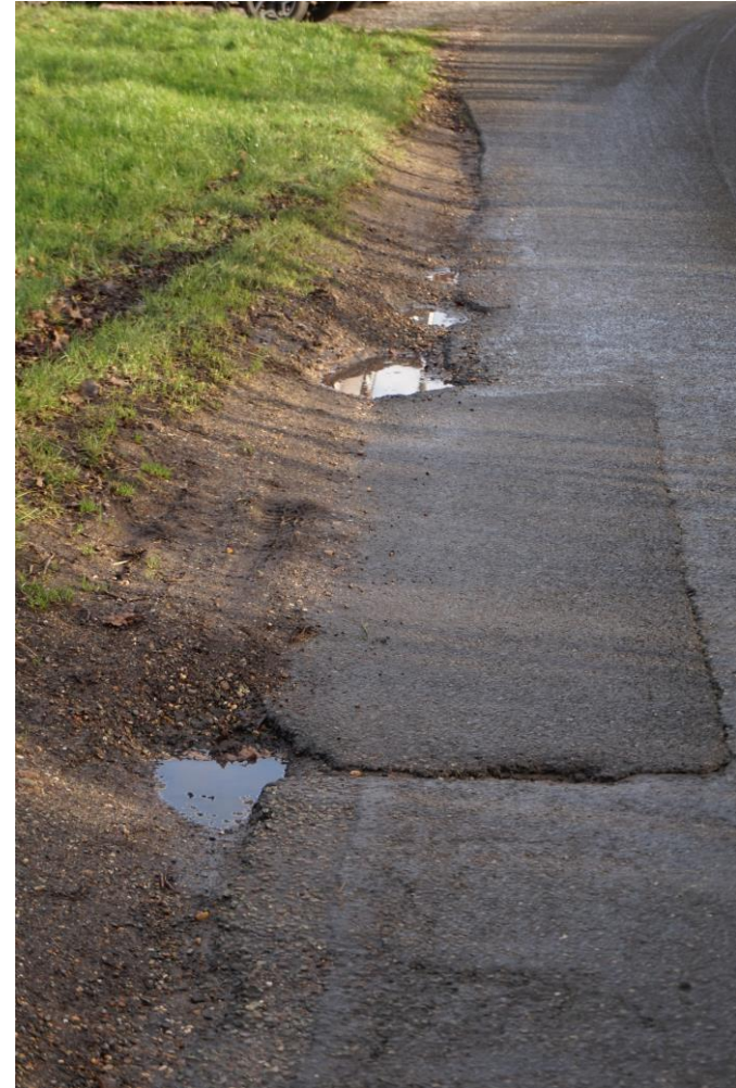
Picture 16 Road damage and verge erosion
