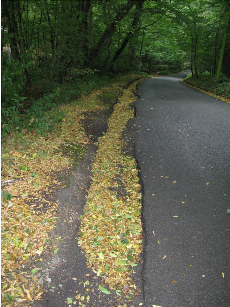
Picture 15 Erosion of verges is being caused by high volumes of traffic trying to pass in narrow lanes
